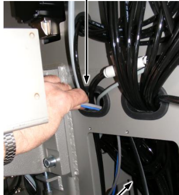
Access Cover Removed
