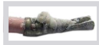
Figure 19. Example of galvanic corrosion on an aluminum wire strand
