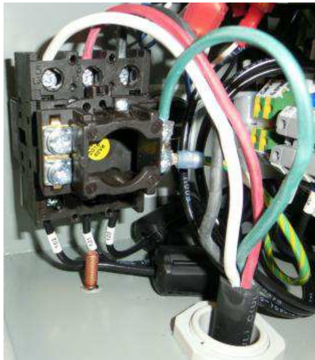
Figure 11: Power disconnect switch
