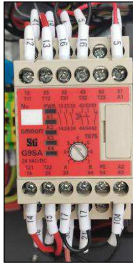
Figure 44: Safety Relay (KS1)
